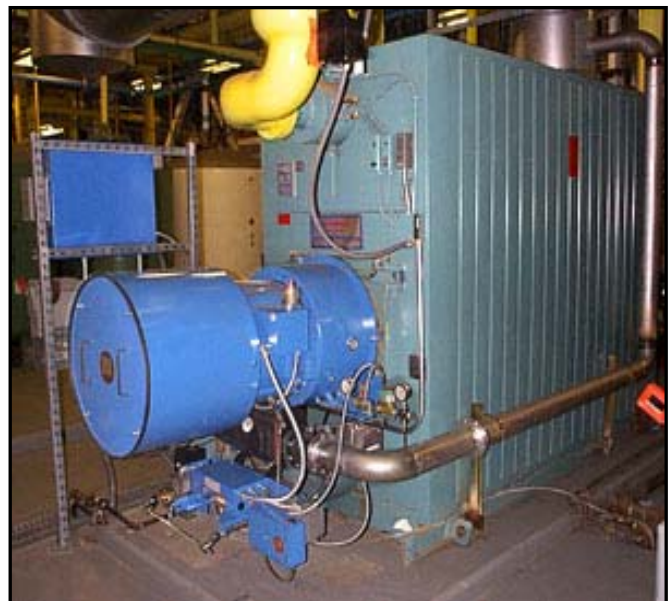
150 HP natural gas & #2 oil flextube boiler application
